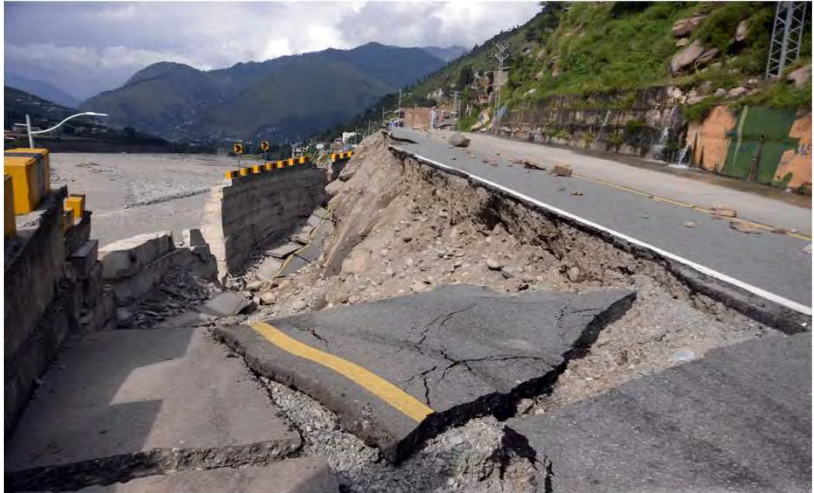
Highway damaged by flood (2022) in Swat, Pakistan
