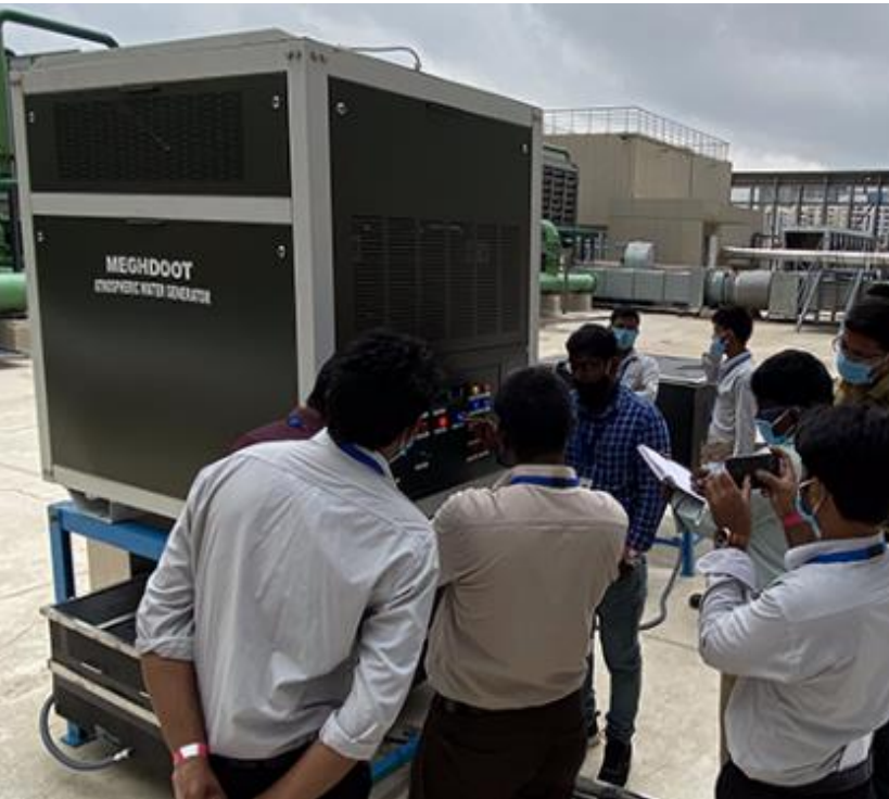
Installation at Amazon, Hyderabad Campus
