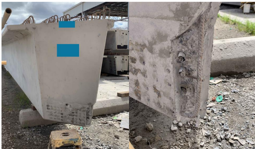
Figure 6 Spalling of acute corner in precast girder unit
