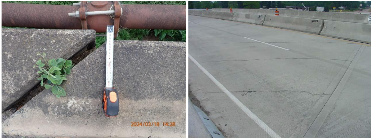
Figure 4: Misalignment at kerb due to transverse movement (L), Corner cracking of skewed concrete bridge (R)
