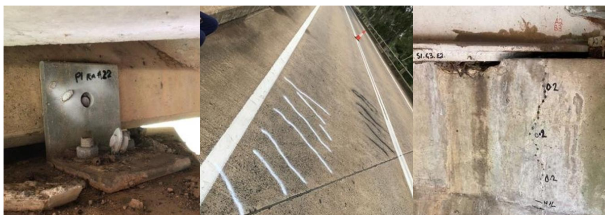
Figure 10: Sheared restraint bolts (L), Deck cracking (M), Abutment cracking (R)
