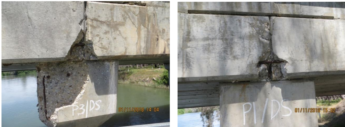
Figure 4 Spalling in planks and pier's headstock at outer faces
