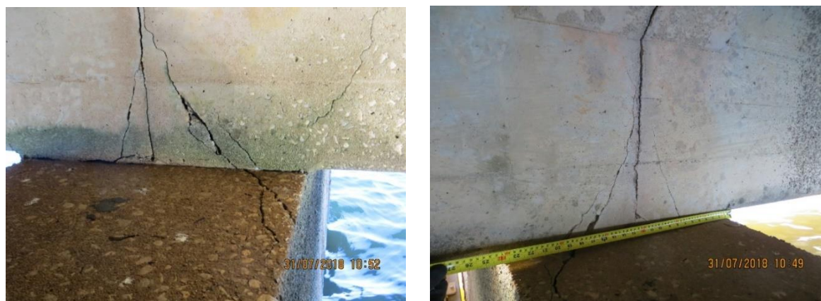
Figure 14 Photos showing crack at the beam ends at the headstock support locations.
