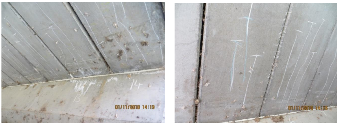
Figure 5 Longitudinal and transverse cracks observed in the plank's soffit of Heywoods Bridge
