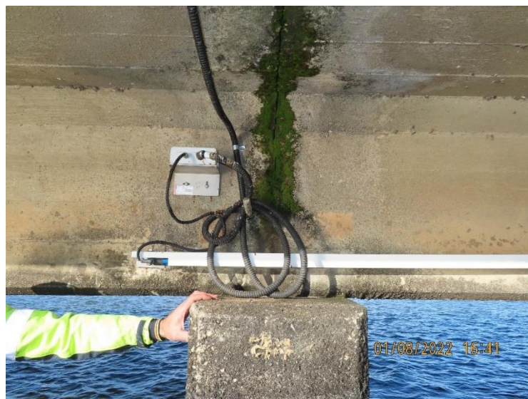
Figure 16 Monitoring system Post installation photo
