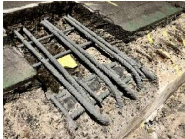
Figure 36 Exposure of rebar and repair
