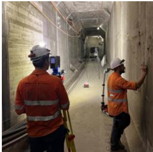
Figure 2 Crack mapping inside a girder
