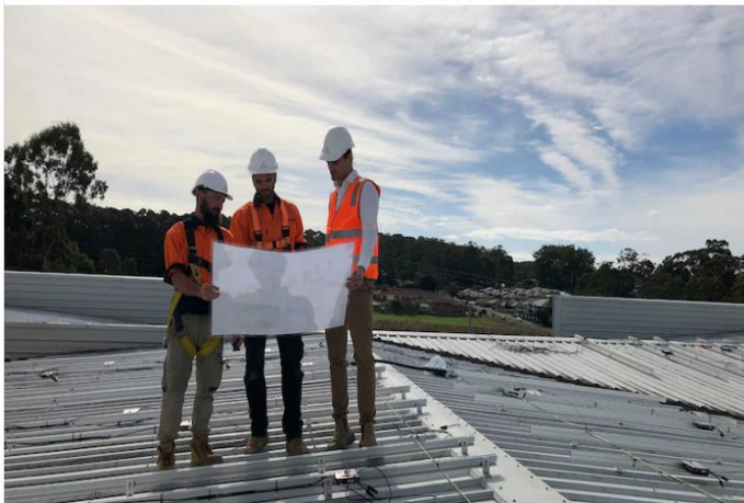
More than 2,000 photovoltaic panels are being installed at the Port Macquarie Base Hospital. (ABC News: Emma Siossian)
