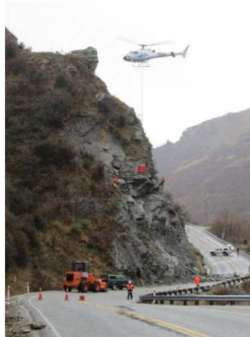
Contractors work to clean and secure the rock face yesterday morning. Photo by James Beech.
