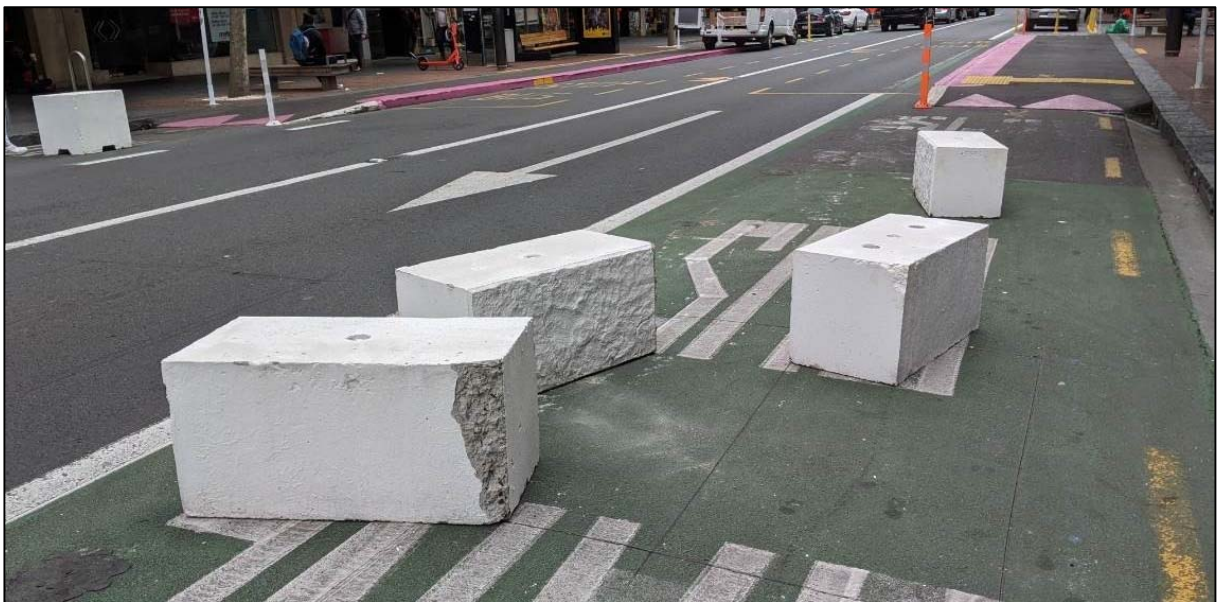
Figure 7: Concrete materials damaged in August 2020
