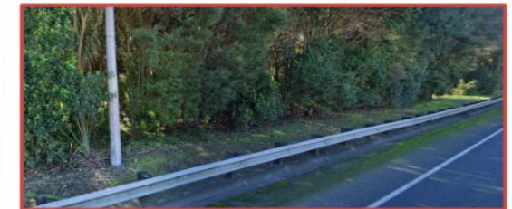
Roadside Guard Rail (W-Beam) Installed in year 2002 (at handover year 2029, asset age = 27) RAMM condition rating in 2023: Poor Recommendation: replacement
