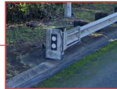
Barrier terminal (M23 Compliant) Installed in year 2002 (at handover year 2029, asset age = 27) RAMM condition rating in 2023: Poor Recommendation: replacement
