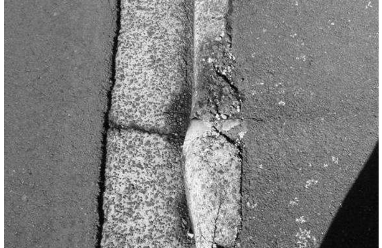
Close up of a curb defect which resulted in an ACC claim
