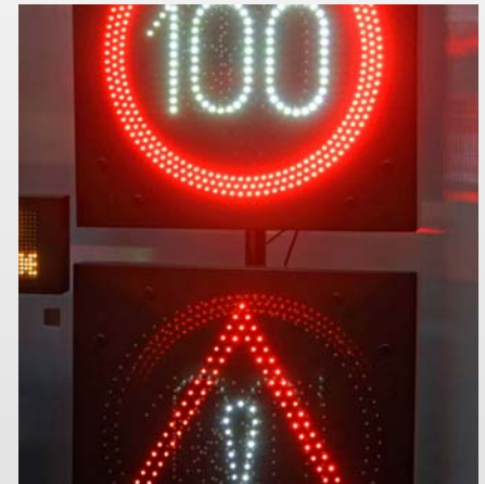
Variable speed limits & lane use signals
