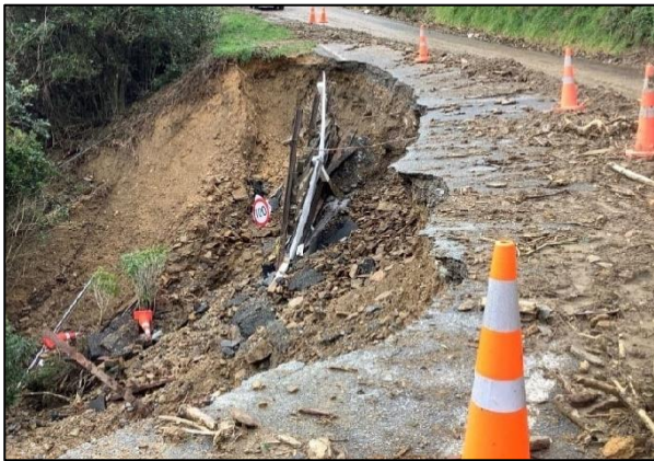
Figure 1: Storm damage from July 2021 on Queen Charlotte Drive, (Marlborough District Council, 2021)
