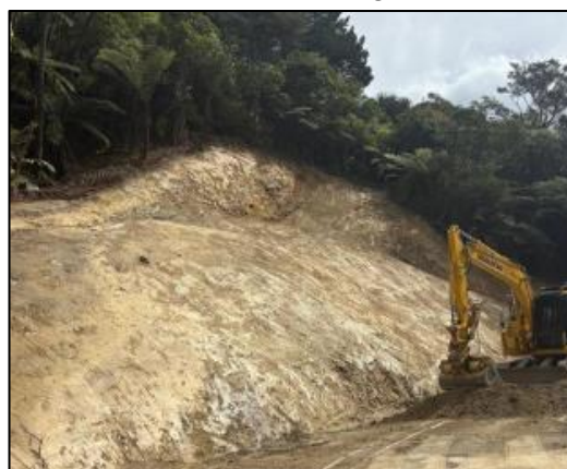
Figure 4: Road retreat solution along Kenepuru Road
