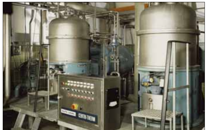
Dual CT-6 units for producing no alcohol beer installed 1984
