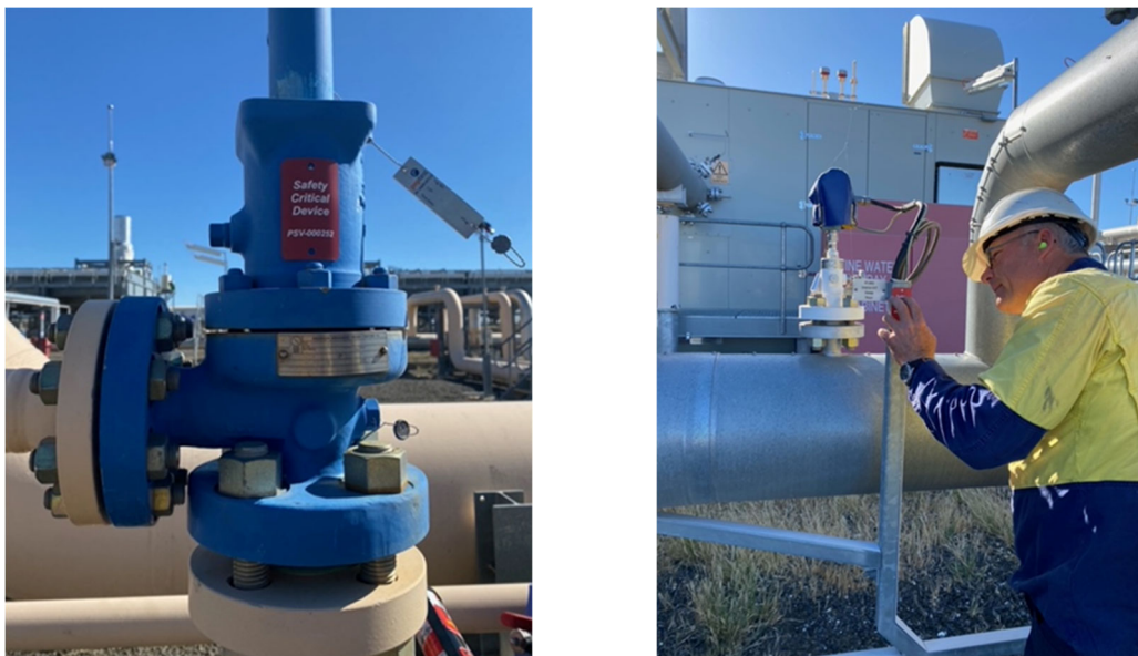
Figure 7: Safety Cruel Device Labelling On-Site
